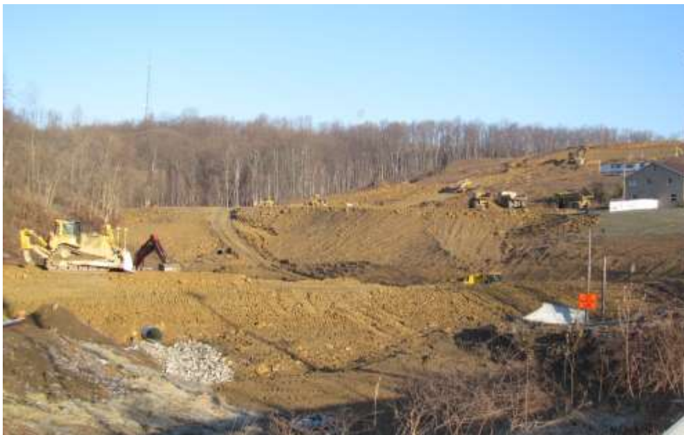
Figure 3. Preparing a Marcellus well site. Photo reprinted with permission from Jeff Skousen, West Virginia University Extension Service.
